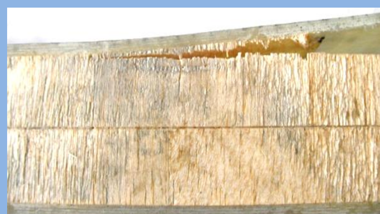
Figure 2: Typical (failed) naval deck sandwich structure (glass fibres and balsa core)
