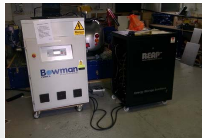
Li-ion Battery Systems and Power Electronics
