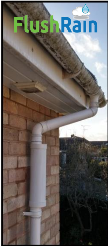
A) Chamber connected to downpipe
